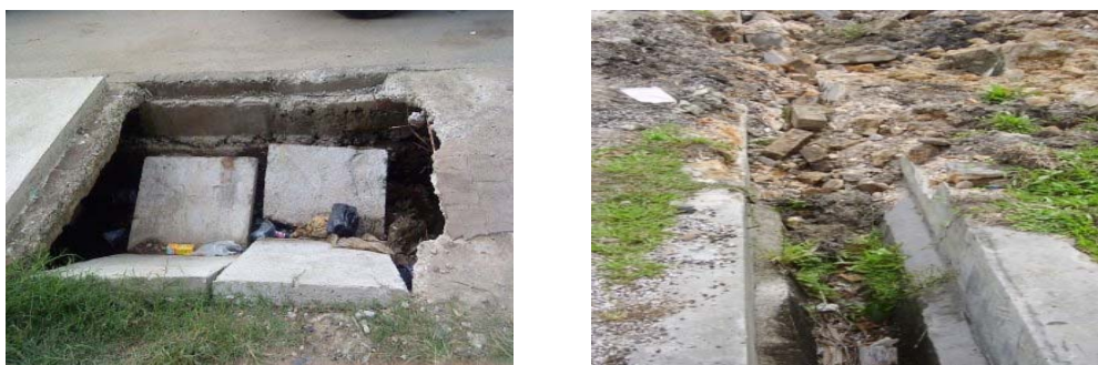
Figure AX2.7: Structure Failure
