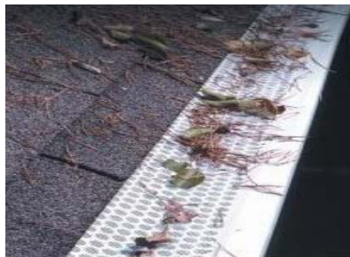
Figure AX2.2: Partially Clogged Gutter Screen
