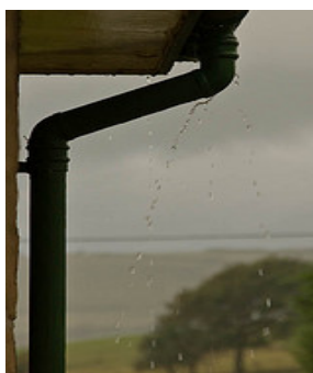
Figure AX2.3: Leaking Downpipe
