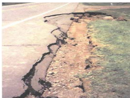
Figure AX2.8: Deterioration of Pavement Edge
