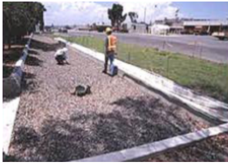
a) Infiltration Trench – Parking lot
