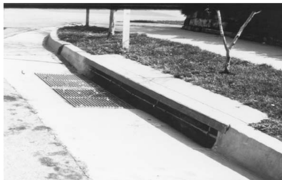
Figure 13.6: Sweeper Combination Inlet
